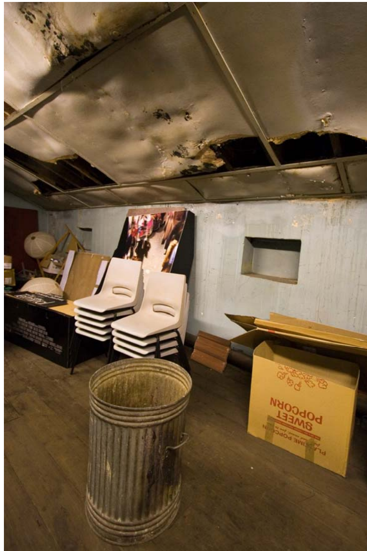
Damage caused by water leaking through the roof
